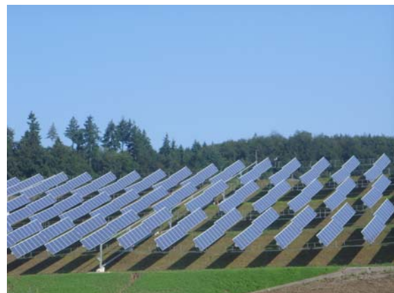
Figure 4: Solar Wings tracking system at the Lonza solar park in Germany.
