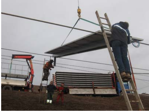
Figure 1: Erecting the Solar Wings tracking system by mounting the pre-assembled eight PV modules onto the supporting cables at the Lonza solar park.
