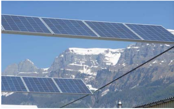
Figure 4: View of the steering cable turning details to rotate the PV plane around the beam carrier axis to follow the daily course of the sun.
