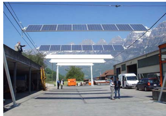
Figure 3: Solar Wings Prototype erected in Flums, Switzerland with a 40m distance between intermediate support pillars. This prototype version is equipped with horizontal PV module axis to allow the utilization of the space below the PV plant as a parking and loading area.
